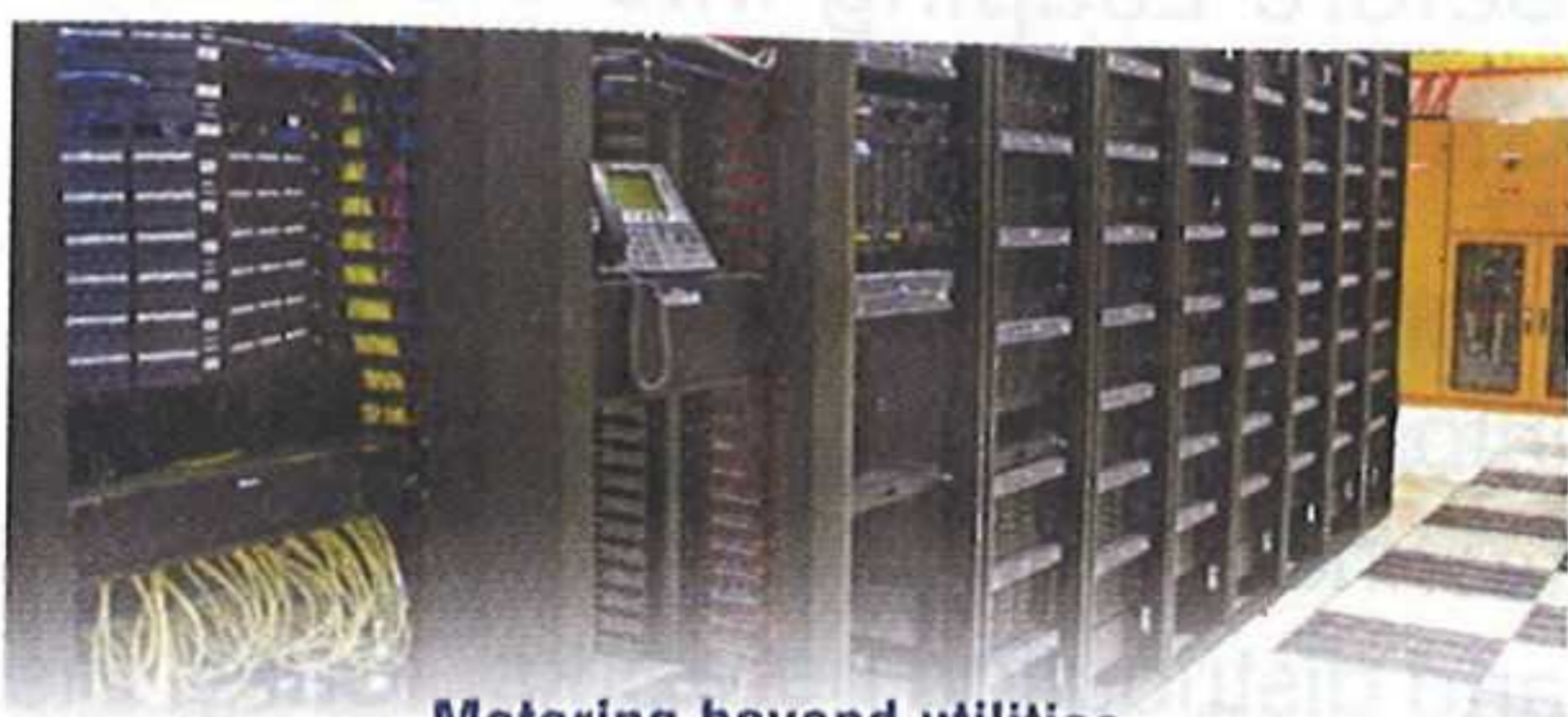
Metering beyond utilities Energy Metering in Data Centers
